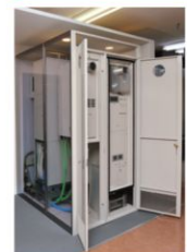
ENE-FARM in an condominium pipe shaft
